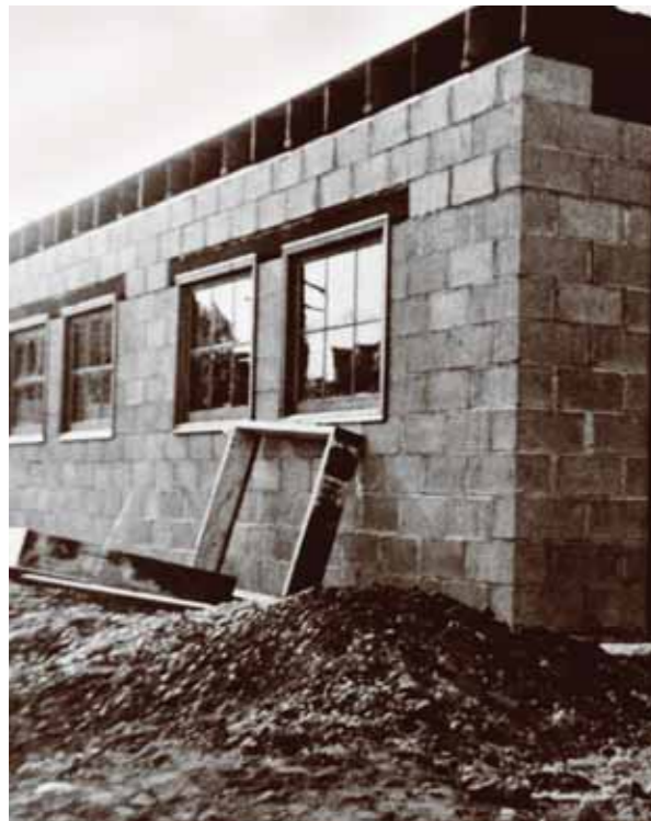
Much of the work on doors and windows in the Marpole workshop was done by Keith and Fred.
